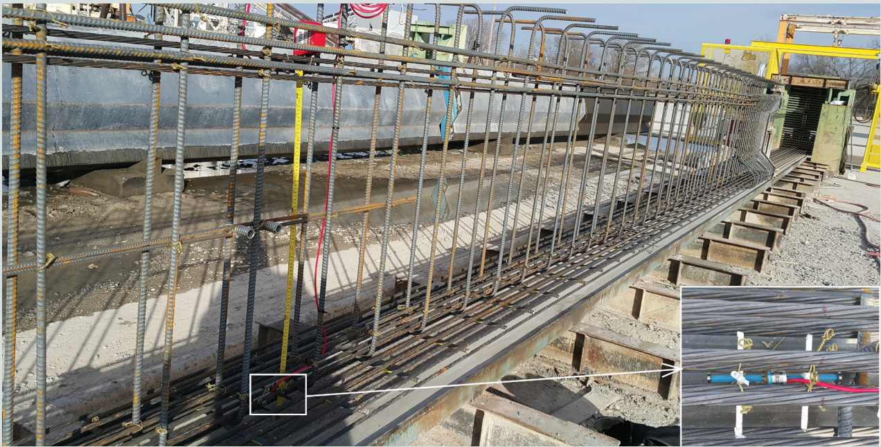
Figure 2. Strain gauges attached to the prestressing strands before installing the side forms.
