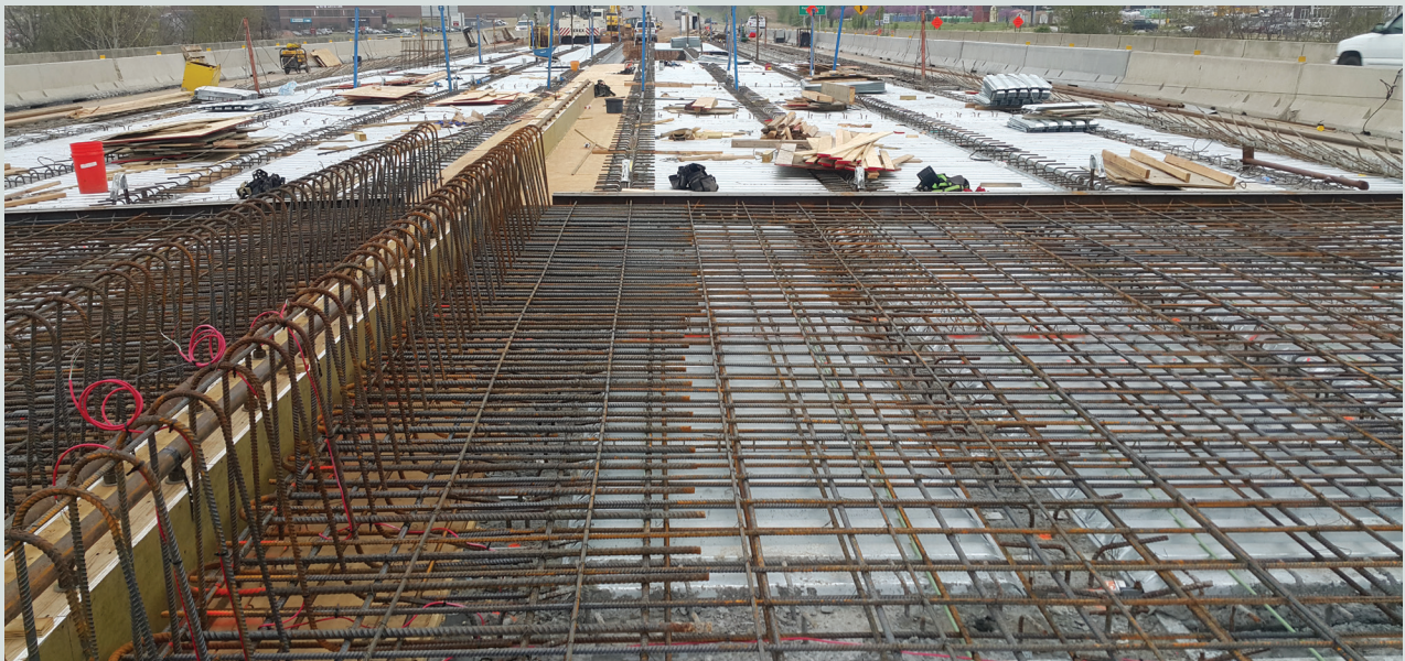
Figure 3. Wires of the strain gauges in the bridge barrier to record the changes in the strands' strain after placing the deck.
